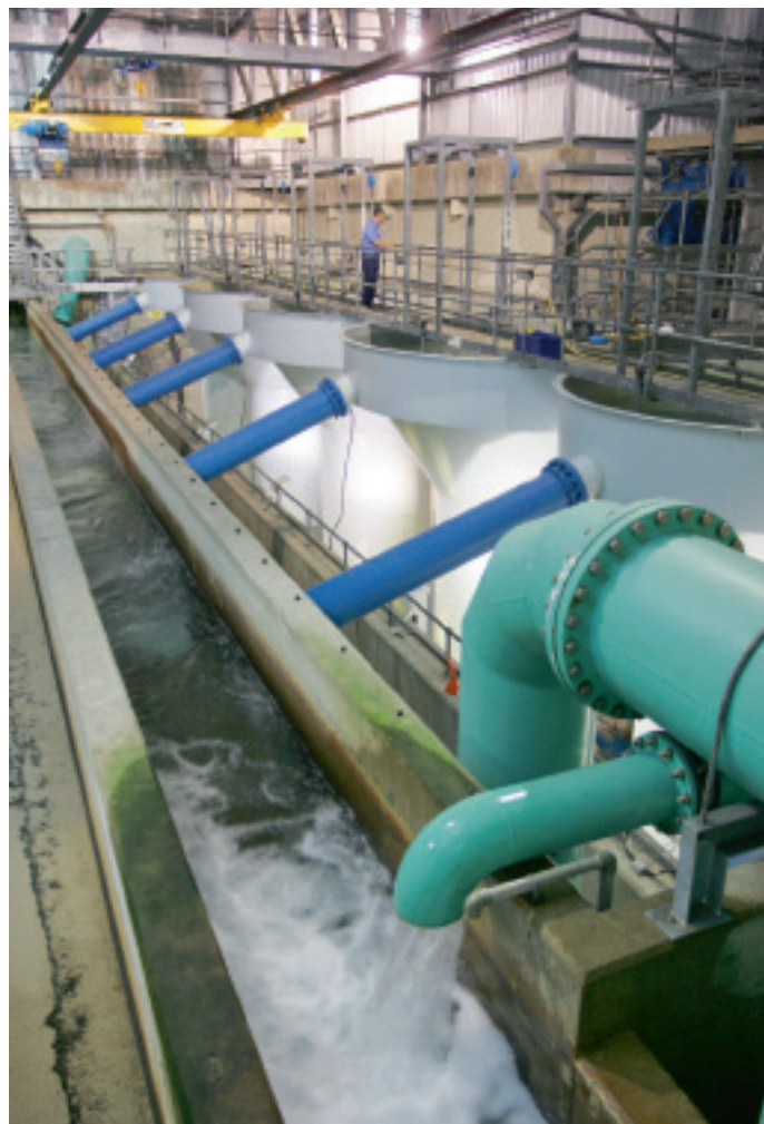
Pictures, above and right, from one of the many modern water treatment works in the South East
